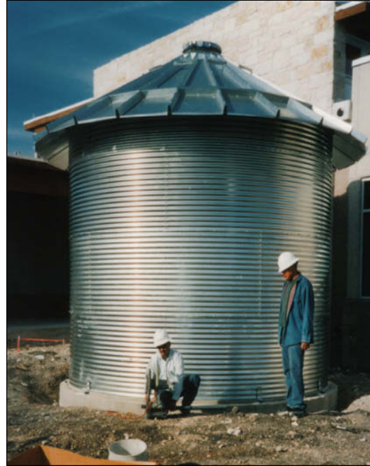
Four lined, galvanized steel tanks will capture water for irrigation of native and adapted plants.
