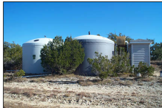
Figure 2-5. Two 10,000-gallon fiberglass tanks
