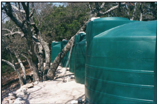
Figure 2-6. Low-profile 5,000-gallon polypropylene tanks
